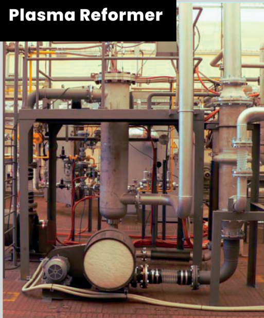
OxEon Plasma Reformer is part of the DAVINCH system for chemical weapons destruction at Kobelco facility in Kanda, Japan.
